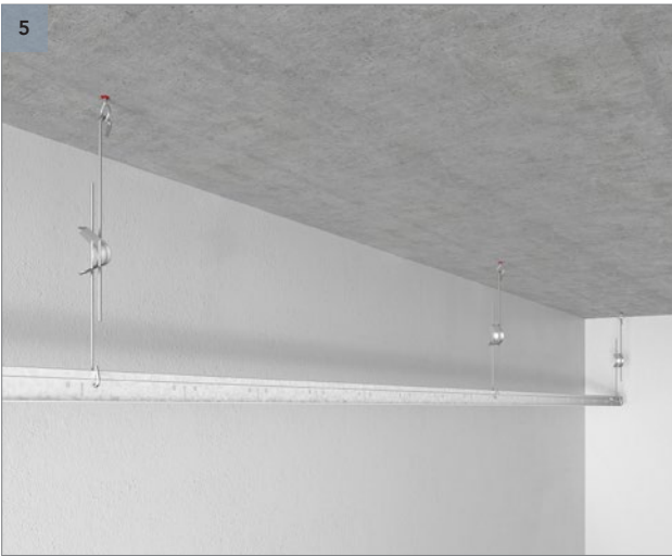
Attach main runner T24 3600 to the bottom of the quick-hangers and remember to secure them by closing the lower hook.
